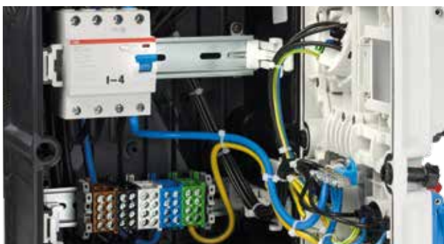
Proper and clearly arranged wiring and an automated safety
